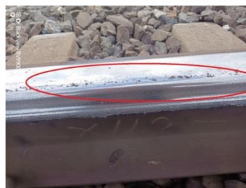
Fig. 2.3. A defect found in curve R = 708 m in Vecumnieki station 1, on the main road.
