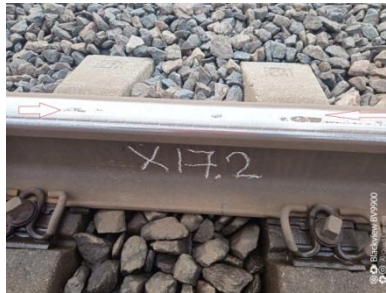
Fig. 2.4. Pitting on rail head surface in Vecumnieki station.
