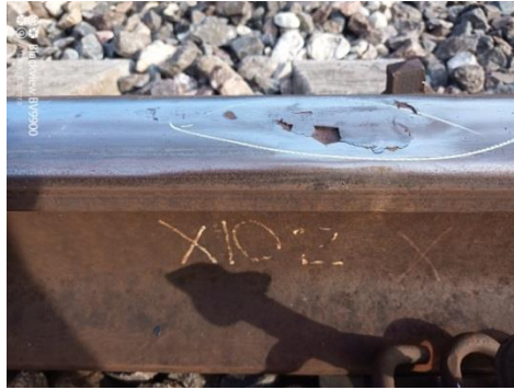
Fig. 2.2. A defect found in rail road section Menta–Daudzeva 256 km 6 pk.
