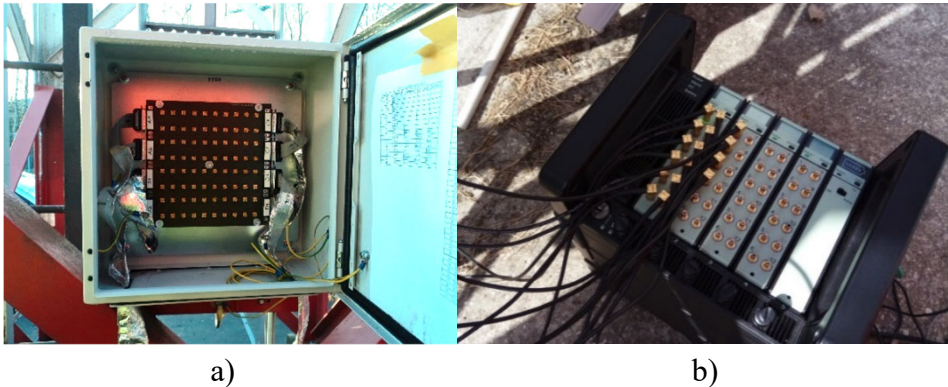
Fig. 4.20. a) Patching panel; b) data acquisition unit.
