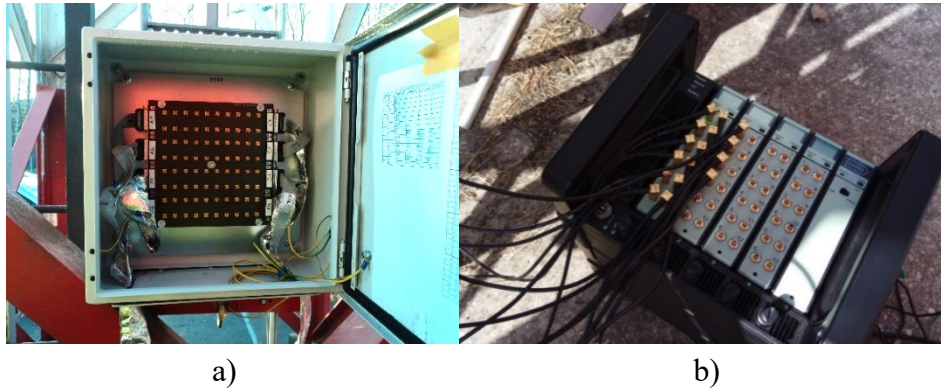
Fig. 4.26. a) Patching panel; b) data acquisition unit.
