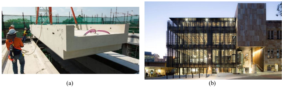
Fig. 10. The Global Change Institute of the University of Queensland building: (a) one of 33 floor panel montage and (b) finished building [170].
