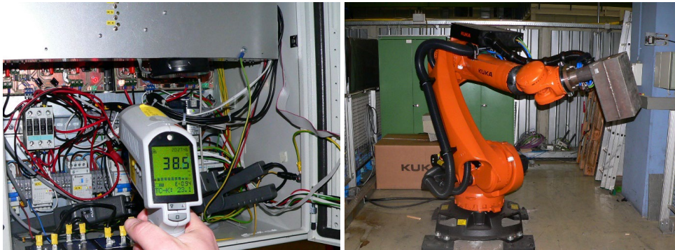
Fig. 2.7. Experimental verification in production area: interconnection module with peripheral devices (left) and one of the interconnected KUKA KR210 industrial robots (right).
