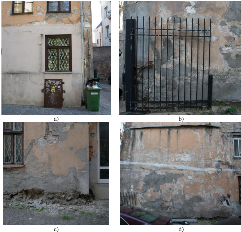
Fig. 3. Façade of the building: a) South-West façade; b) South corner; c) right corner of South-East façade; d) South-East façade.
