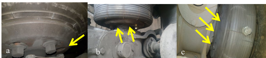
Fig. 3.27. Rubber-cord coupling degradation patterns: a – fracture of the 1st bolt; b – two bolt fractures; c – three bolt fractures.
