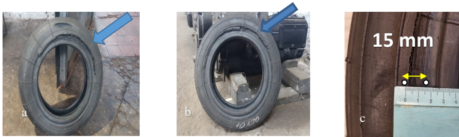
Fig. 3.1. Examples of the side surface disintegration of a rubber-cord coupling: a – sample 1; b – sample 2; c – determining the destruction zone sample 2.
