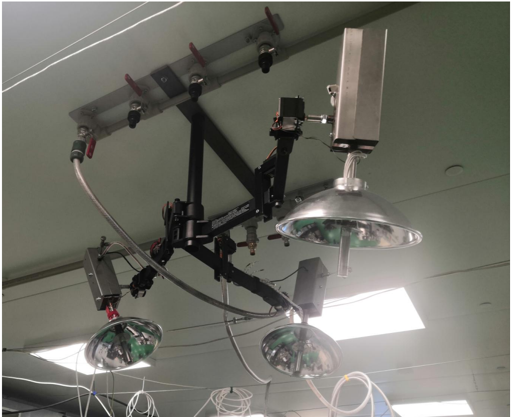
Figure 5-6. Ceiling lighting system composed of three HLP-based LED luminaires with independent positioning.
